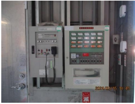
Fire alarm system
